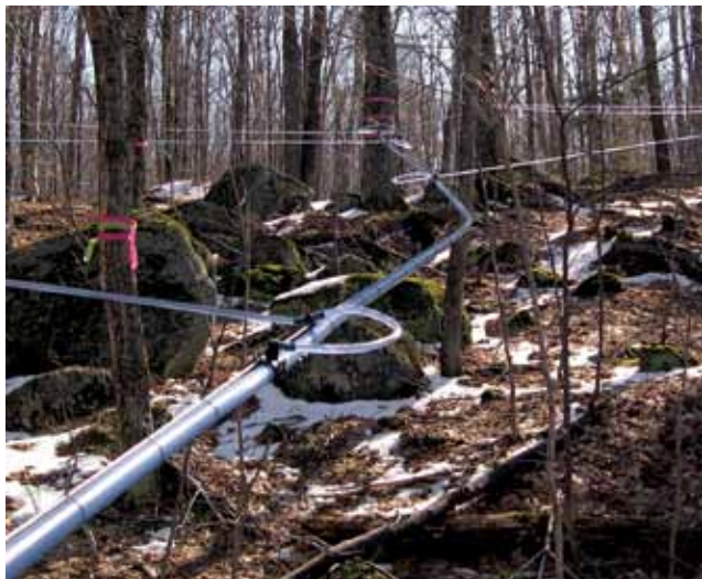
Figure 6.10. Tubing systems should be designed so gravity helps sap move through the system. When properly installed, tubing is tight, straight, and sloping downhill.
