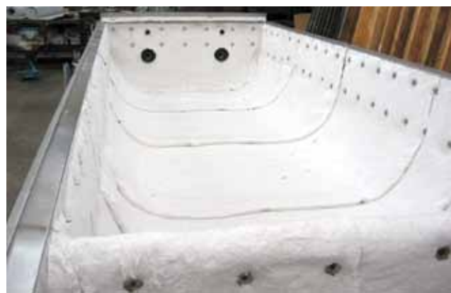
Figure 7.13. Oil and gas fired evaporators use a ceramic blanket to insulate the arch.
