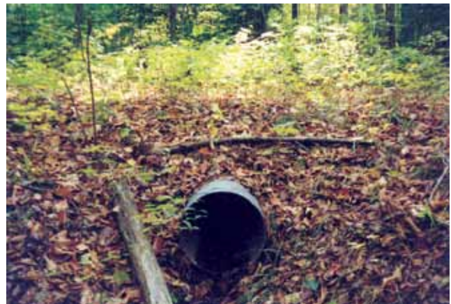
Figure 5.37. Closed culverts are conduits that move water from one side of the road to the other without it flowing on the road surface. A closed culvert would be used, for example, to move water from a drainage ditch on the up-slope side of a road to the down-slope side.
