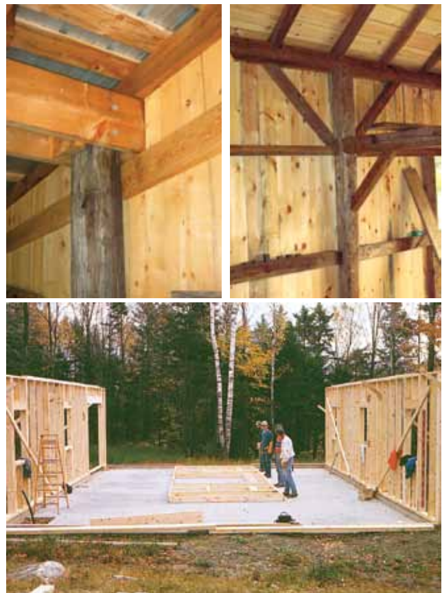
Figure 12.3. Construction methods commonly used when building a sugarhouse include post-frame or pole barn (upper left), post-and-beam (upper right), and light frame (bottom).
