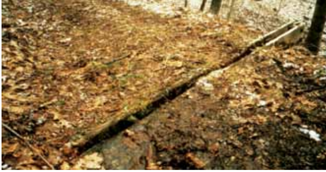
Figure 5.36. Open top culverts are structured openings at a down-slope angle across a road that intercept water and carry it off the road. Notice that this culvert demonstrates a lack of adequate maintenance—open top culverts need to be periodically cleaned.
