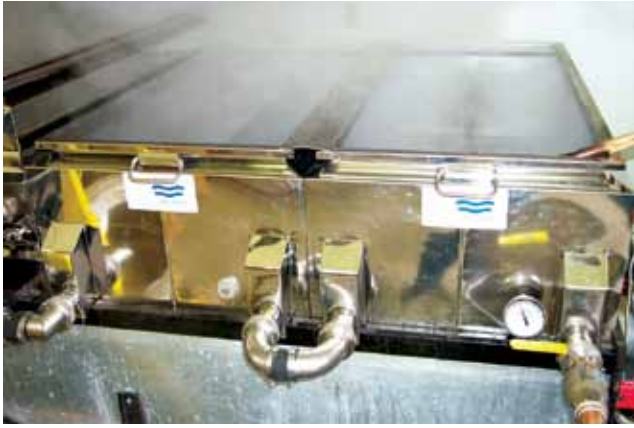
Figure 7.7. Pipe connecting cross flow syrup pans.
