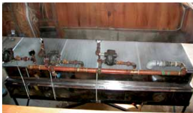
Figure 7.19. Steam evaporators. Notice in the lower evaporator that the parallel steam pipes are visible in the bottom of the evaporator pan.
