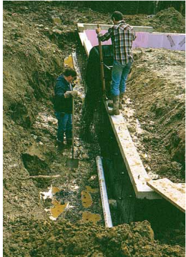
Figure 12.4. Increasing the amount of gravel and adding perforated pipe and curtain drains to control ground and surface moisture will help to prevent frost damage to the slab.
