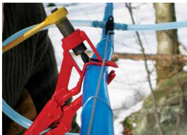
Figure 6.25. Mainline punch used to drill hole in mainline when installing saddle fitting.
