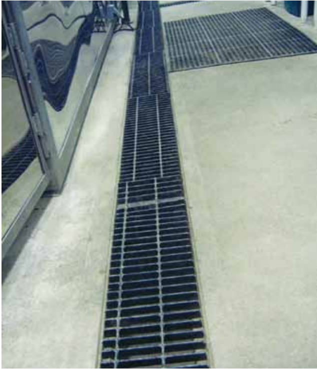
Figure 12.6. Adequate floor drainage in the sugarhouse might include a drain running the length of the evaporator or one running around the perimeter of the evaporator.
