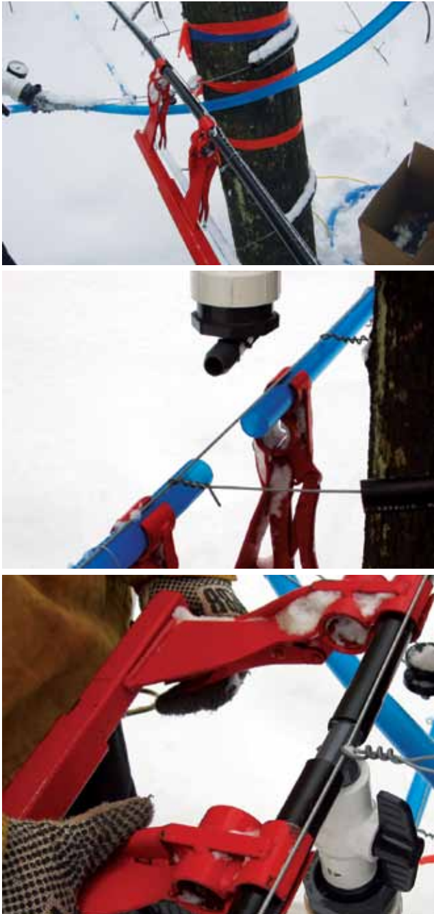
Figure 6.20. Mainline installation tool, which grips the tubing and holds it in place while it is cut, then pushes the tubing over both sides of the fitting by turning a crank that closes the tool.
