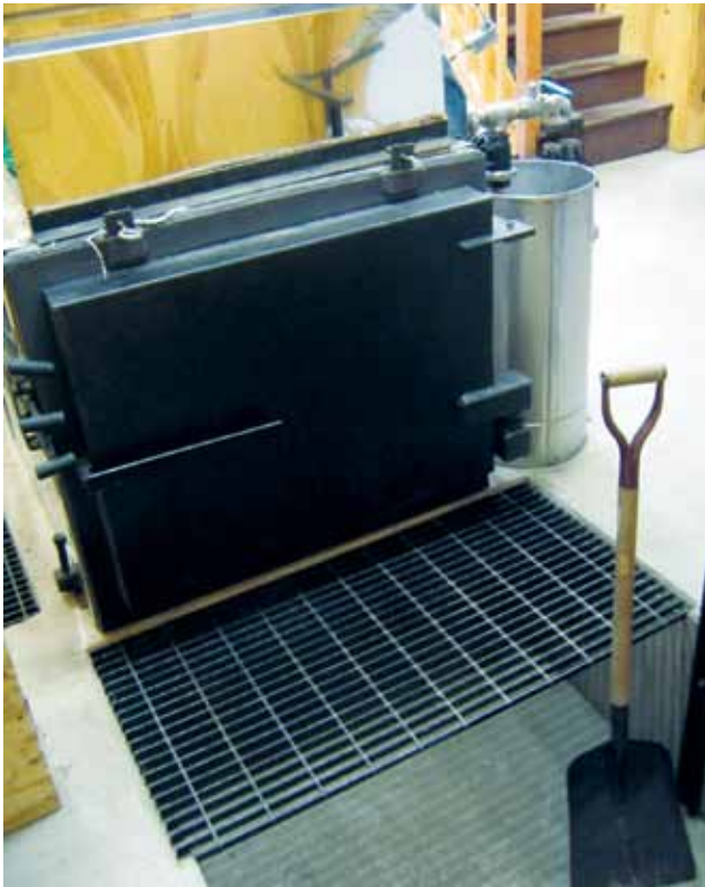
Figure 12.7. Incorporating a recessed pit in the floor in front of the firebox is a convenient feature in a wood-fired operation.
