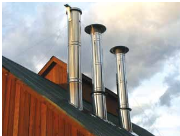
Figure 12.10. Steam stacks venting water vapor from evaporator.
