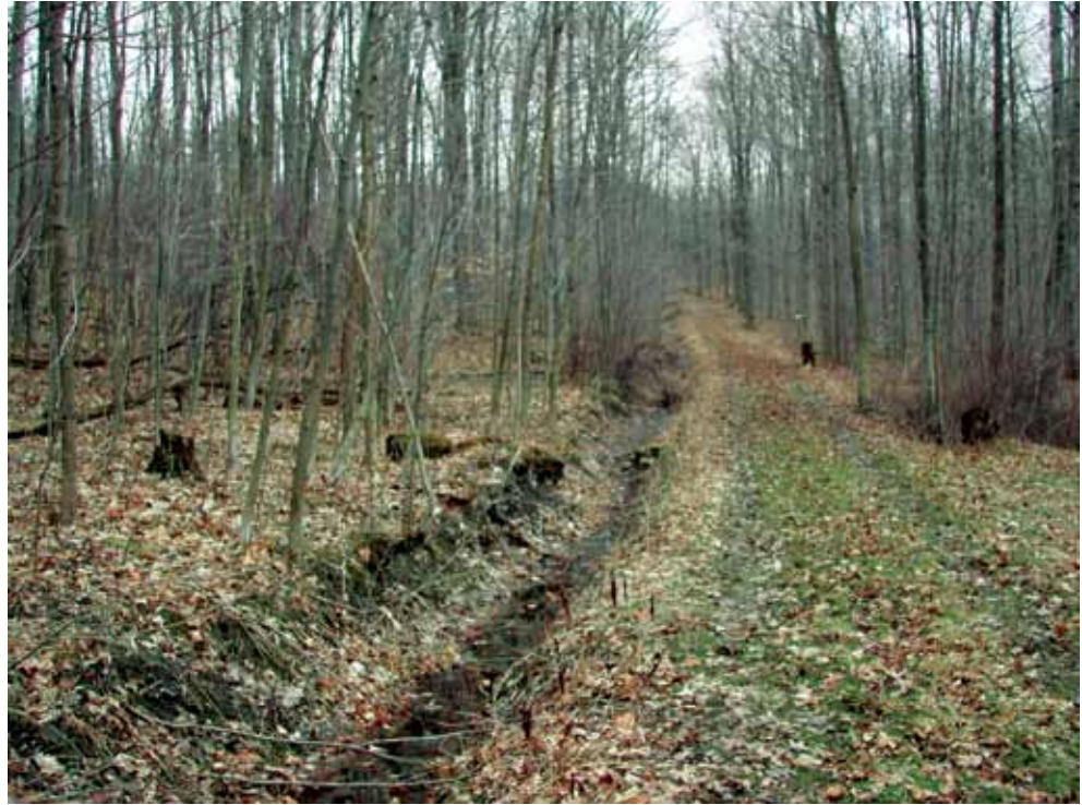
Figure 5.33. An example of an acceptable sugarbush road. The road has a ditch on the uphill side, is crowned and slightly sloped to the downhill side, and enough light is currently available to maintain vegetative cover on the road.
