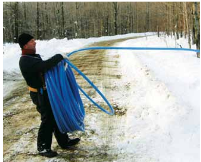
Figure 6.17. The most effective way to distribute mainline in the woods is generally to pull the free end while the coil is unrolled by a helper.
