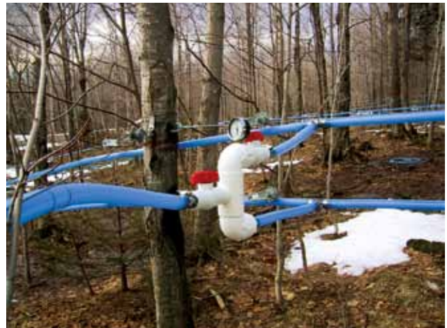
Figure 6.26. Manifold connecting lateral mainline to vacuum (upper) and sap (lower) lines in a dual conductor or wet line/dry line tubing system.
