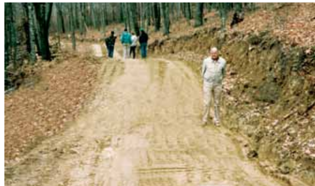
Figure 5.35. A broad-based dip is a low, relatively flat, out-sloped diversion in the roadbed designed to intercept water flowing down the roadbed and drain it to the side, off the road surface.
