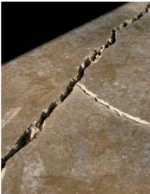
Figure 12.5. Pouring concrete on an inadequately prepared base can result in cracking.
