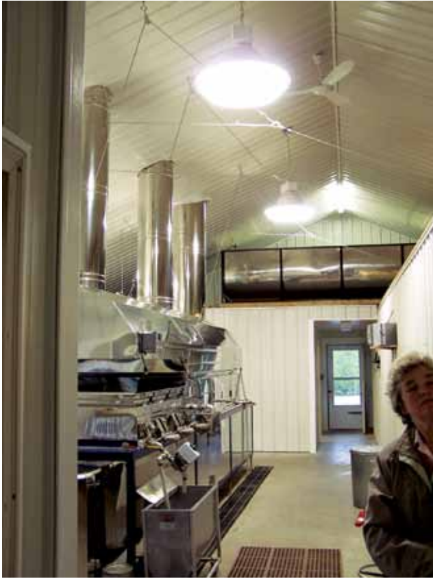
Figure 12.13. Cables attached to collar ties can be used to relieve stress on the evaporator from the weight of a “Piggyback” or “STEAM-AWAY®.”
