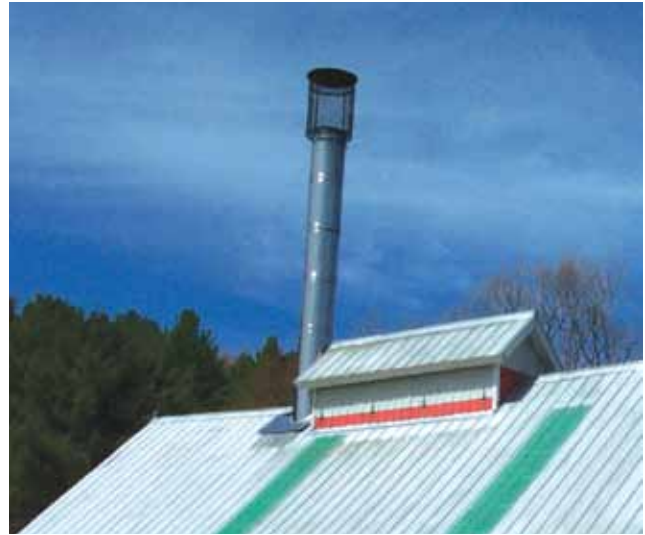
Figure 12.12. A spark arrester is useful in preventing release of these potential fire starters.
