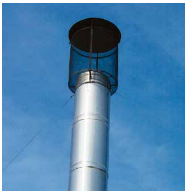
Figure 13.7. Spark arrester on top of smoke stack.
